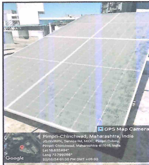
Photograph of Roof Top Solar PV Plant:
